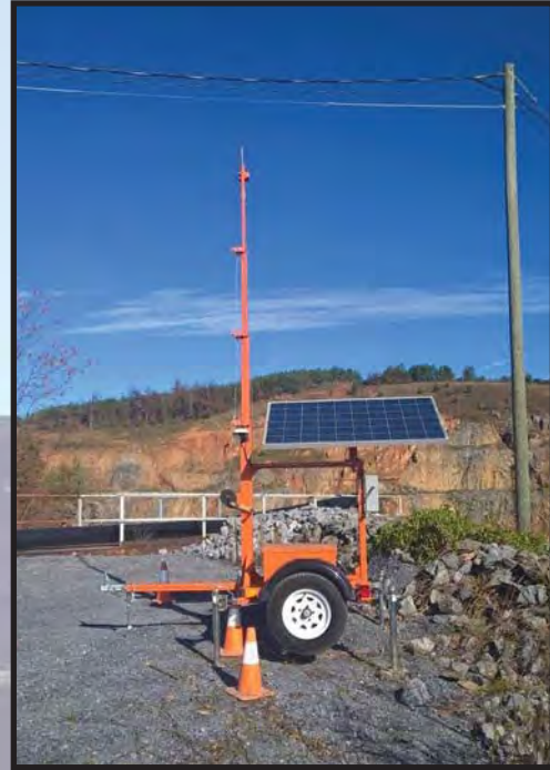
Solar Powered Wi-Fi Repeater & GPS Base Station
